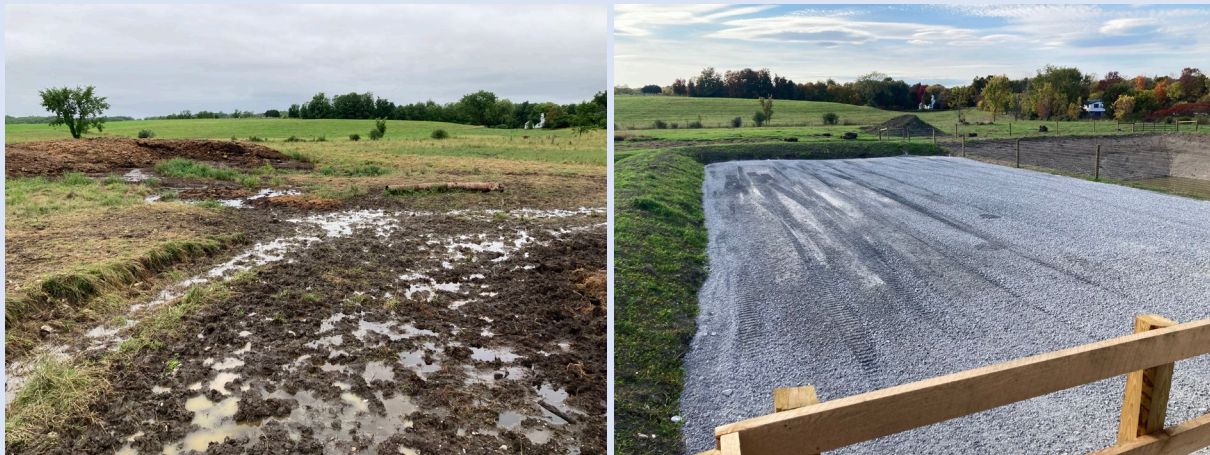
Figure 3. Before (left) and after (right) installation of a new waste storage facility and adjacent solid manure stack site.
