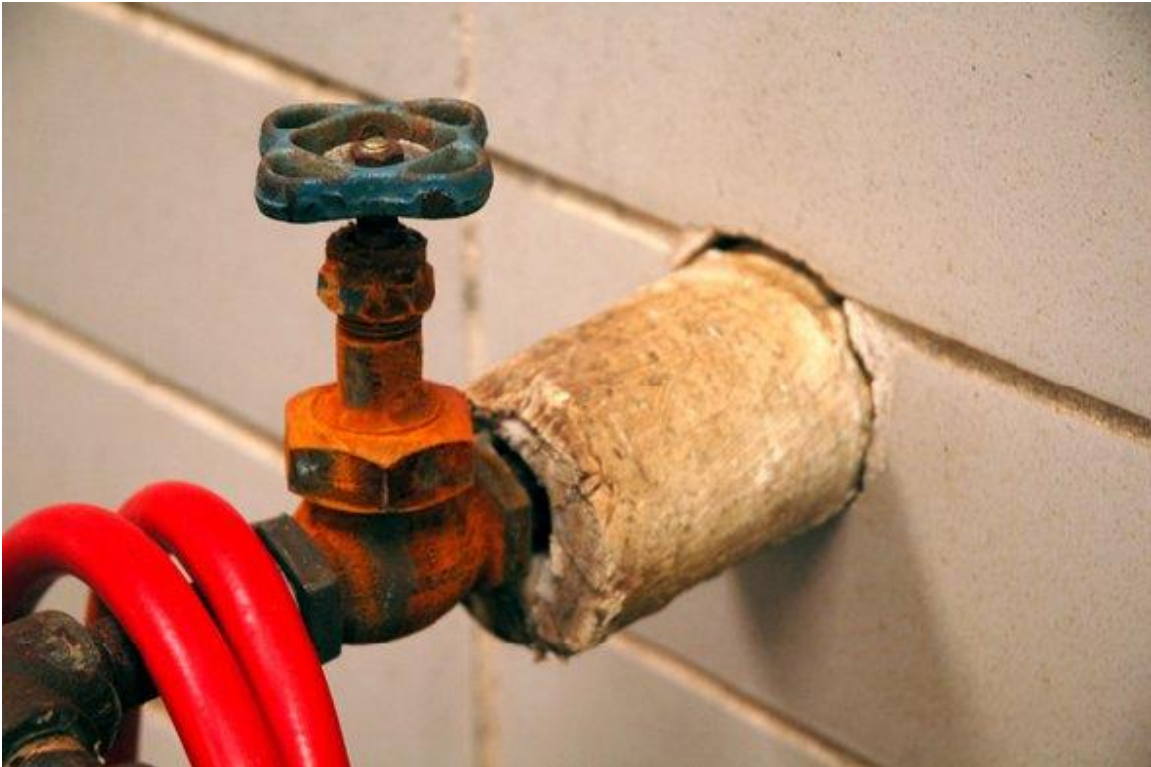
A rusty water spigot with a dirty, cracked insulated pipe. Lm could spread to the hose and be sprayed in the establishment.
