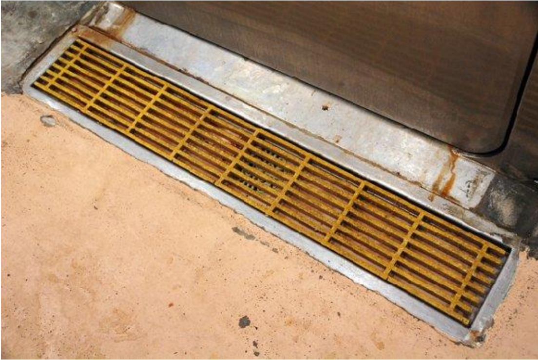
A drain at the entrance of a cooler doorway. The drain could become contaminated with Lm , and when employees step on the drain to enter the cooler, the Lm can spread into the cooler.
