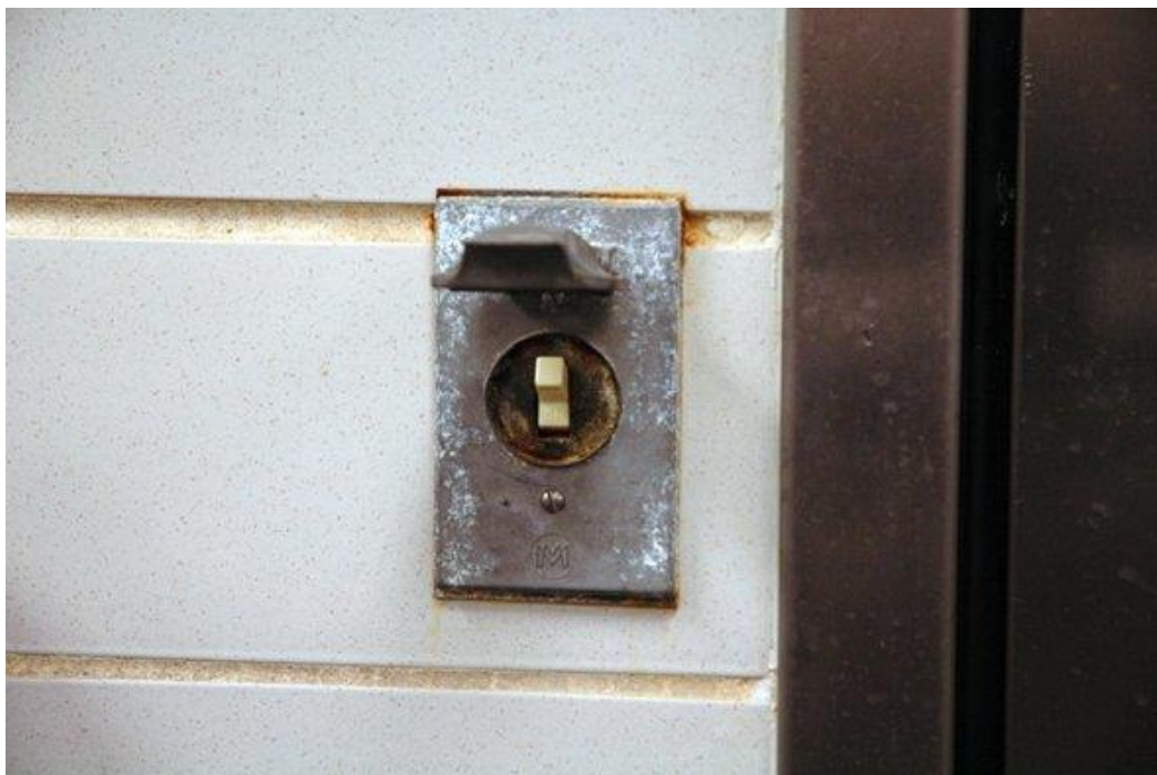
A light switch with residue build-up and grime. The switch could be contaminated with Lm by employees' hands during operation, and may not be cleaned during sanitation. When the light is turned on the next day, the hands could be re-contaminated.
