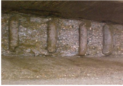
Raised cement cleats on alley ramp
