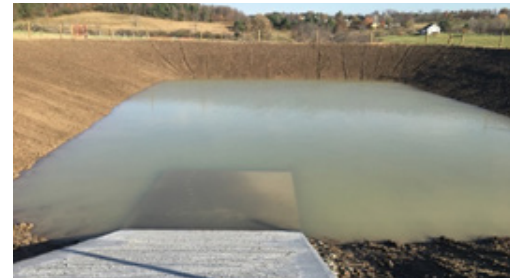
Above - Waste Storage Facility implemented voluntarily on a beef CSFO in Benson through Vermont's BMP Program. Below - Clean Water Project Sign displayed adjacent to farm sign during
