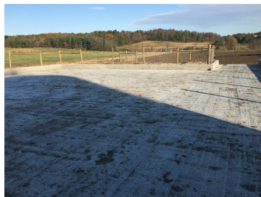
From top to bottom, implemented Waste Storage Facility and Heavy Use Area on a CSFO in Benson
