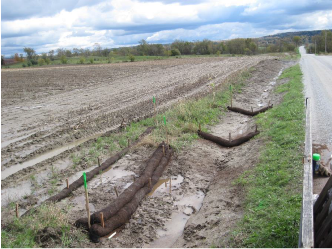
Filter Sock used at buffer breach to trap nutrients and sediment before they reach ditch. Slow flow in ditch to aid infiltration and reduce erosion.
