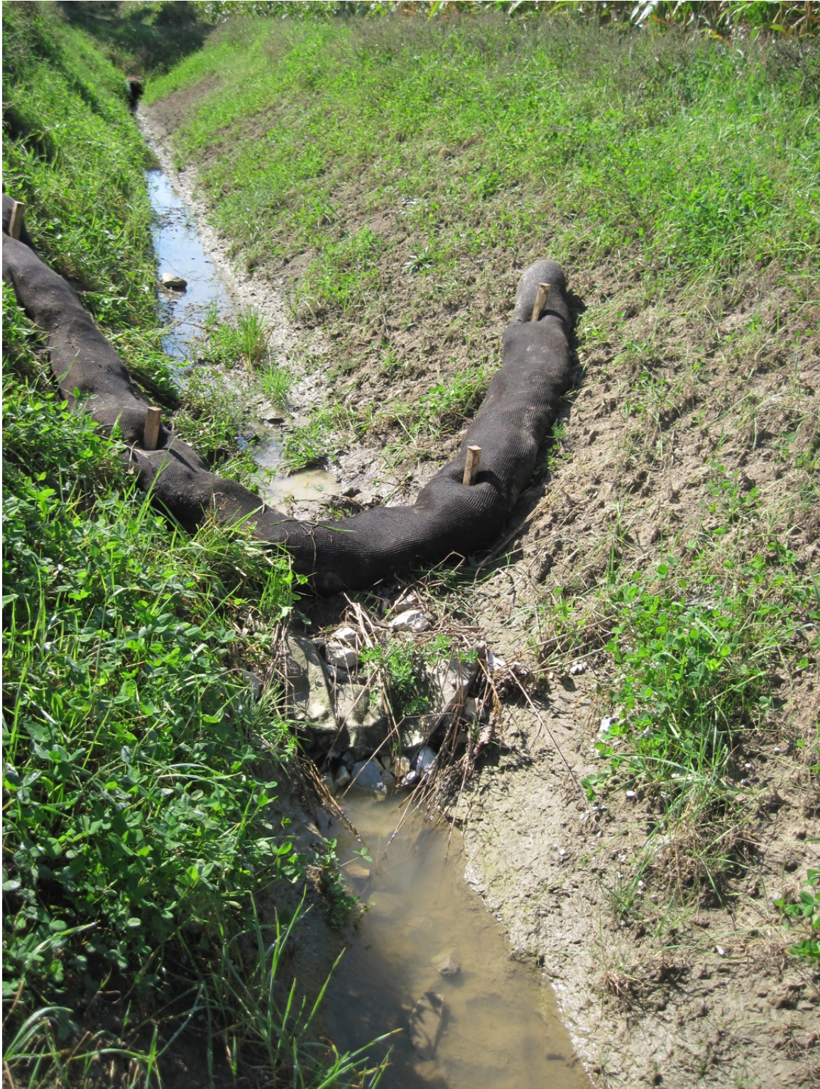
Ditch walls too steep with unstable, eroding soil. Slow flow to aid infiltration
