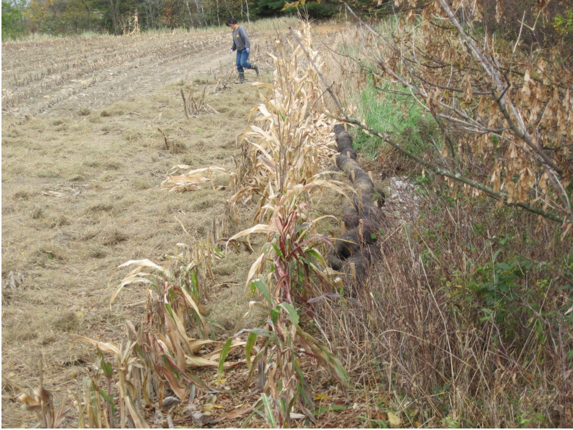
Compost Filter Sock installed above check dam. Adjacent field area seeded and covered with mulch hay.
